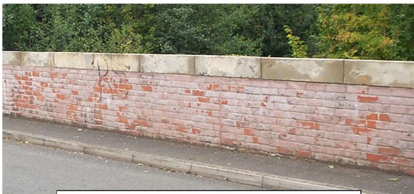
Unsuccessful anti-graffiti coating on a bridge in Leicestershire.
