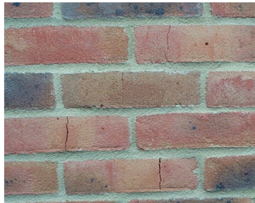
Fire-cracks in clay brick. Cracks do not extend into the mortar joint suggesting their presence when built in.
