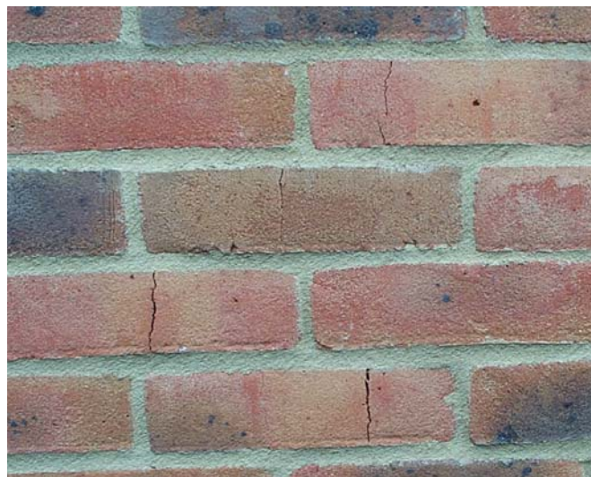
Firecracks in clay brick. Cracks do not extend into the mortar joint suggesting their presence when built in.
