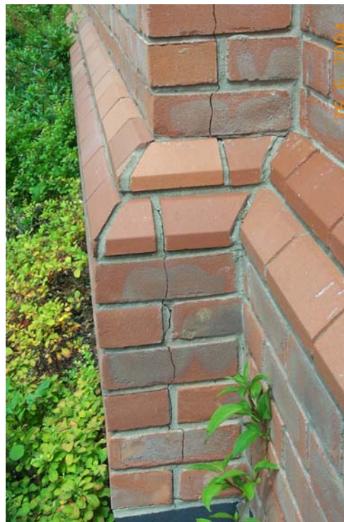
Inadequate provision for movement causing cracking in a short return.
